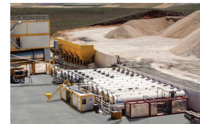
TURKEY - modIFALT 40 PMB Plant up to 40 t/h
